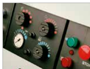
CONTROL PANEL PROVIDED WITH EMERGENCY SHUTDOWN
